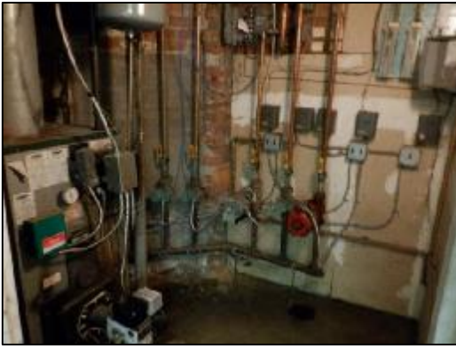
Interior, As-Is – basement, hot water boiler
