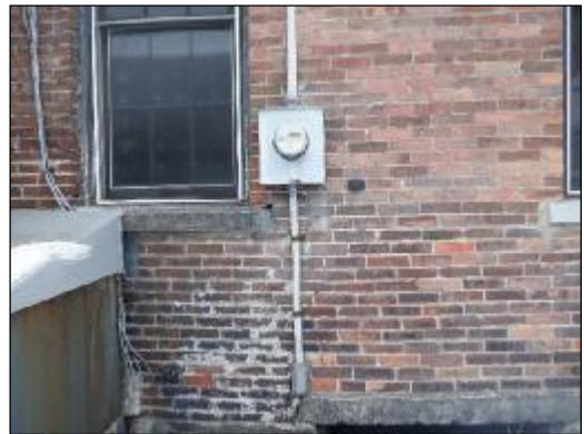
Exterior, As-Is – electrical service
